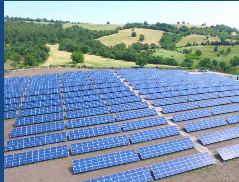
1 MW SOLAR POWER PLANT PROJECT CANAKKALE
